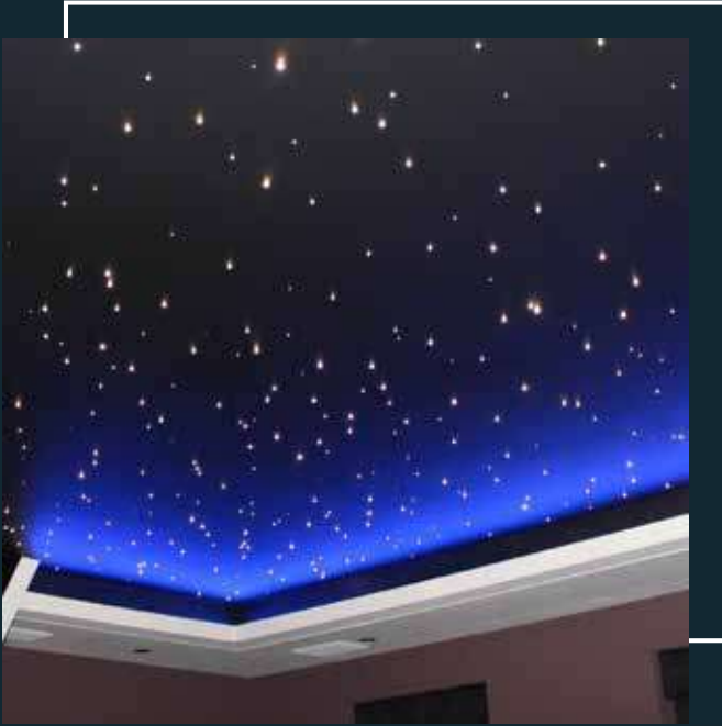
Ceiling Fiber Optics
